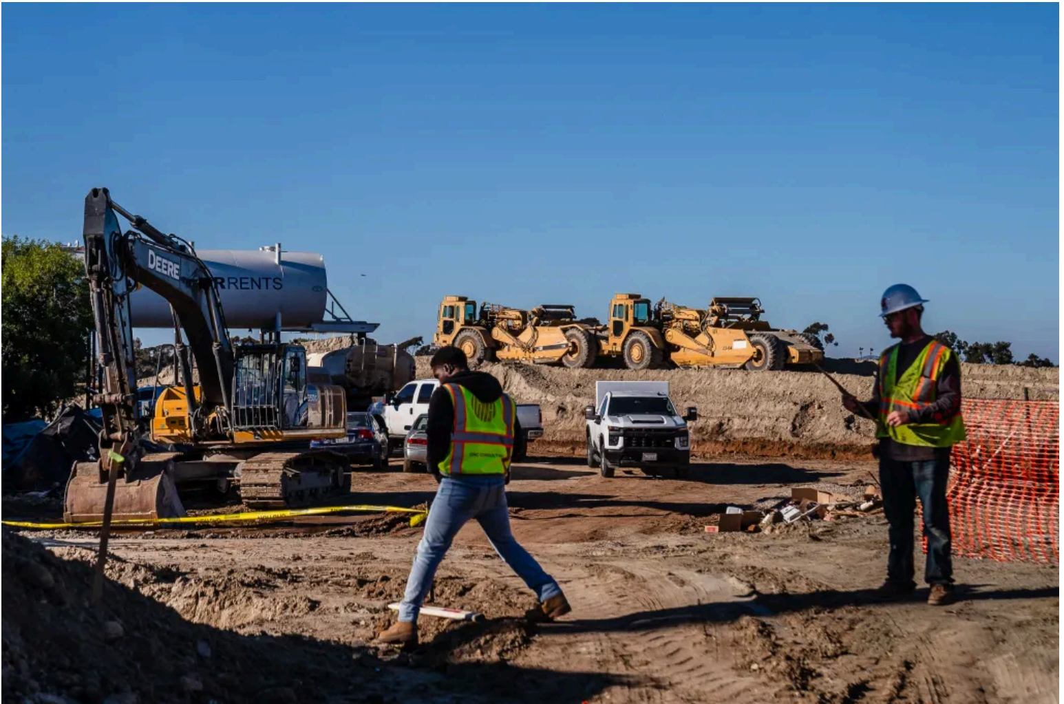
A housing development being built in Oceanside on Dec. 8, 2022. / Photo by Ariana Drehsler
