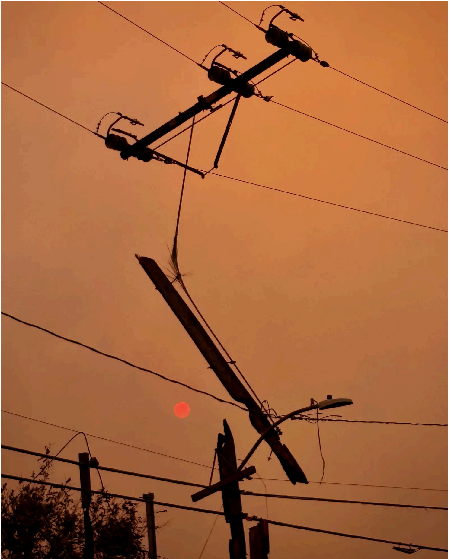
A telephone pole burned through by the Eaton Fire, in Altadena.
